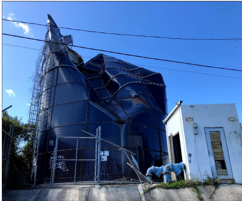
Damaged water tank from winds of Hurricane Maria observed in February 2020
