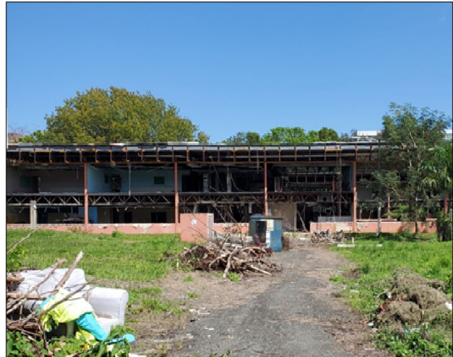
School observed in March 2022 awaiting repairs. According to a FEMA official, a construction crew removed doors, windows, and some walls due to asbestos and lead in the building.
