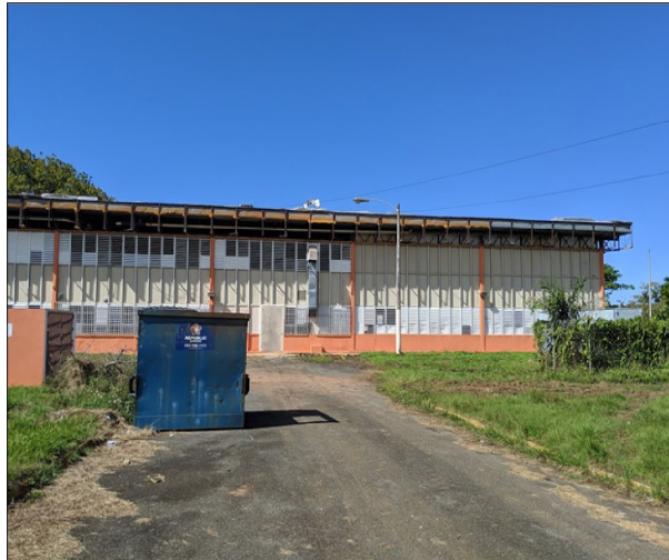
School with internal mold and water damages caused by Hurricane Maria observed in March 2019.
