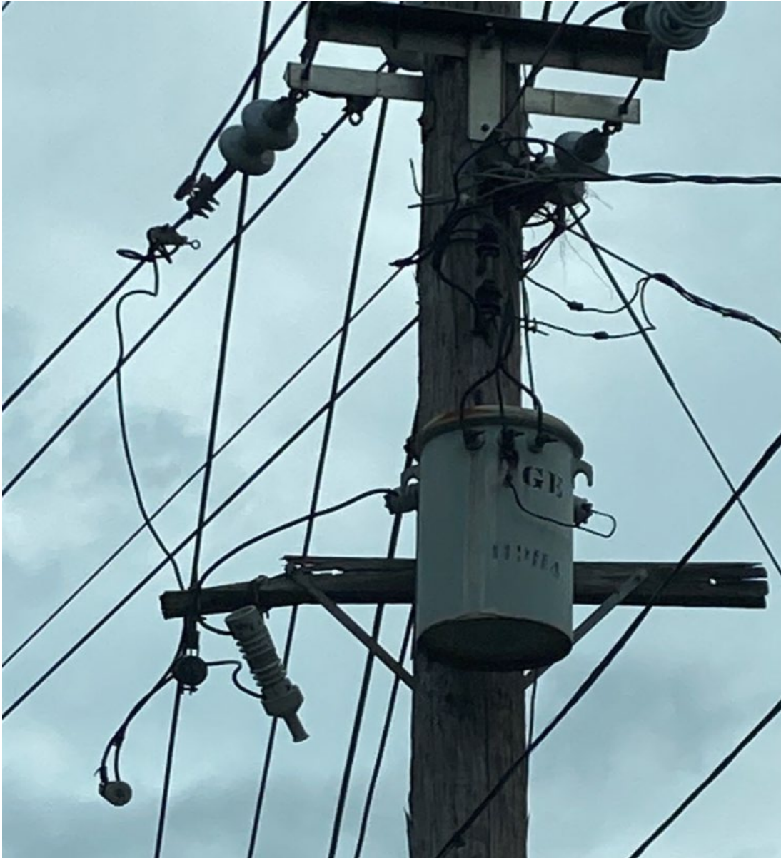
Failed cross arm. Poor workmanship.
