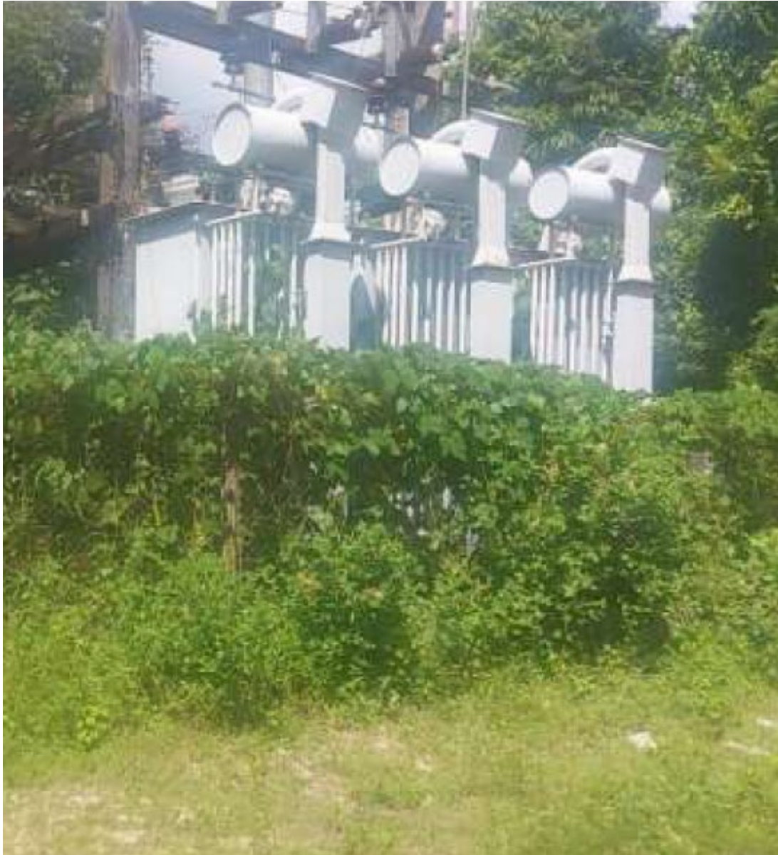
Substation overgrown with vegetation.
