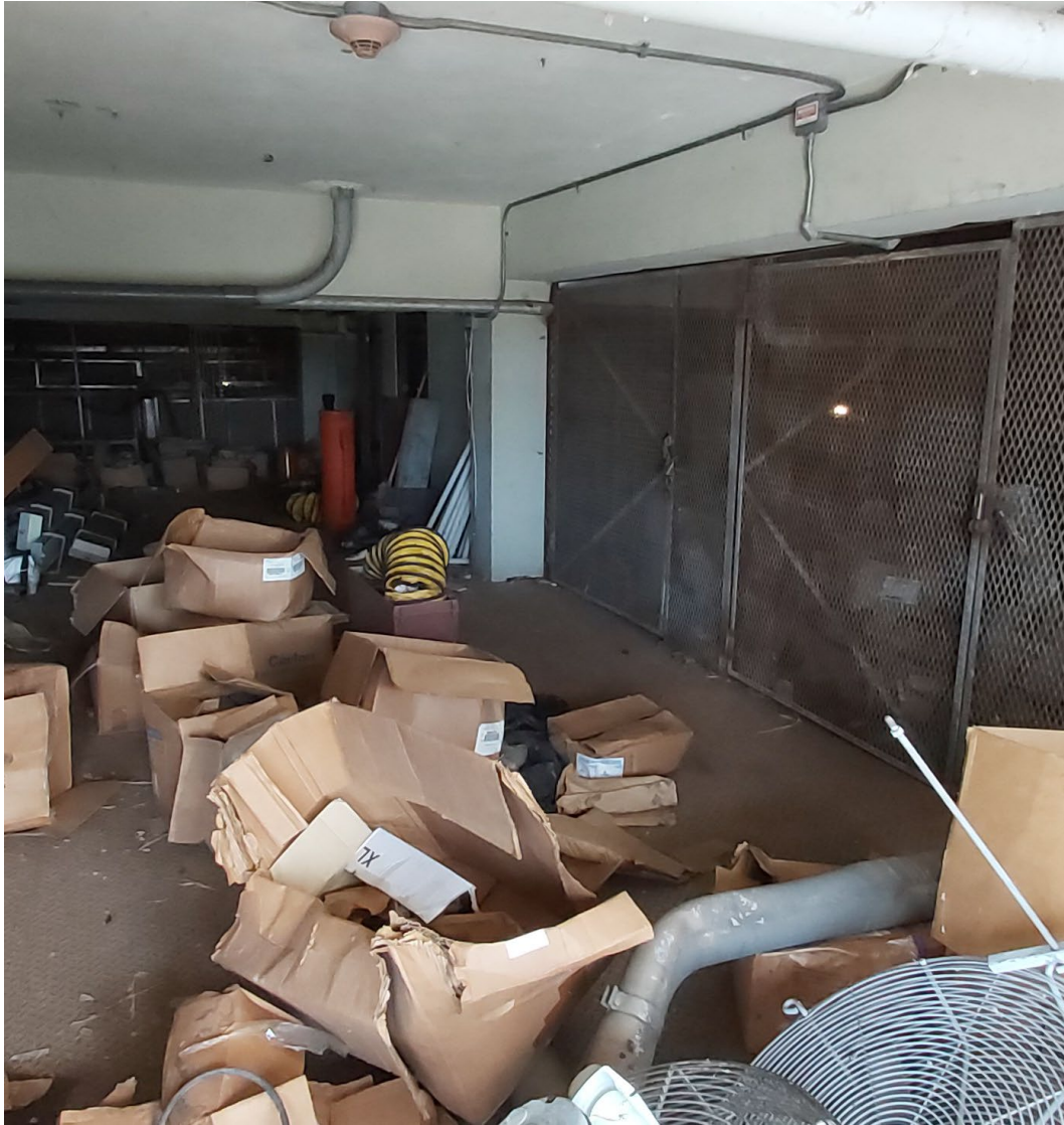
Monacillo Durex building - Rat infested storage of scrap material - still being raided for parts.
