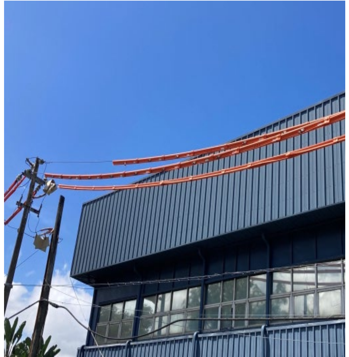
37 piece of line cover up 3 blankets beach from sun no repairs.
