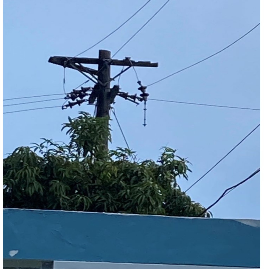
Failed cross arm. Failed hardware. Primary laying in cross arm.
