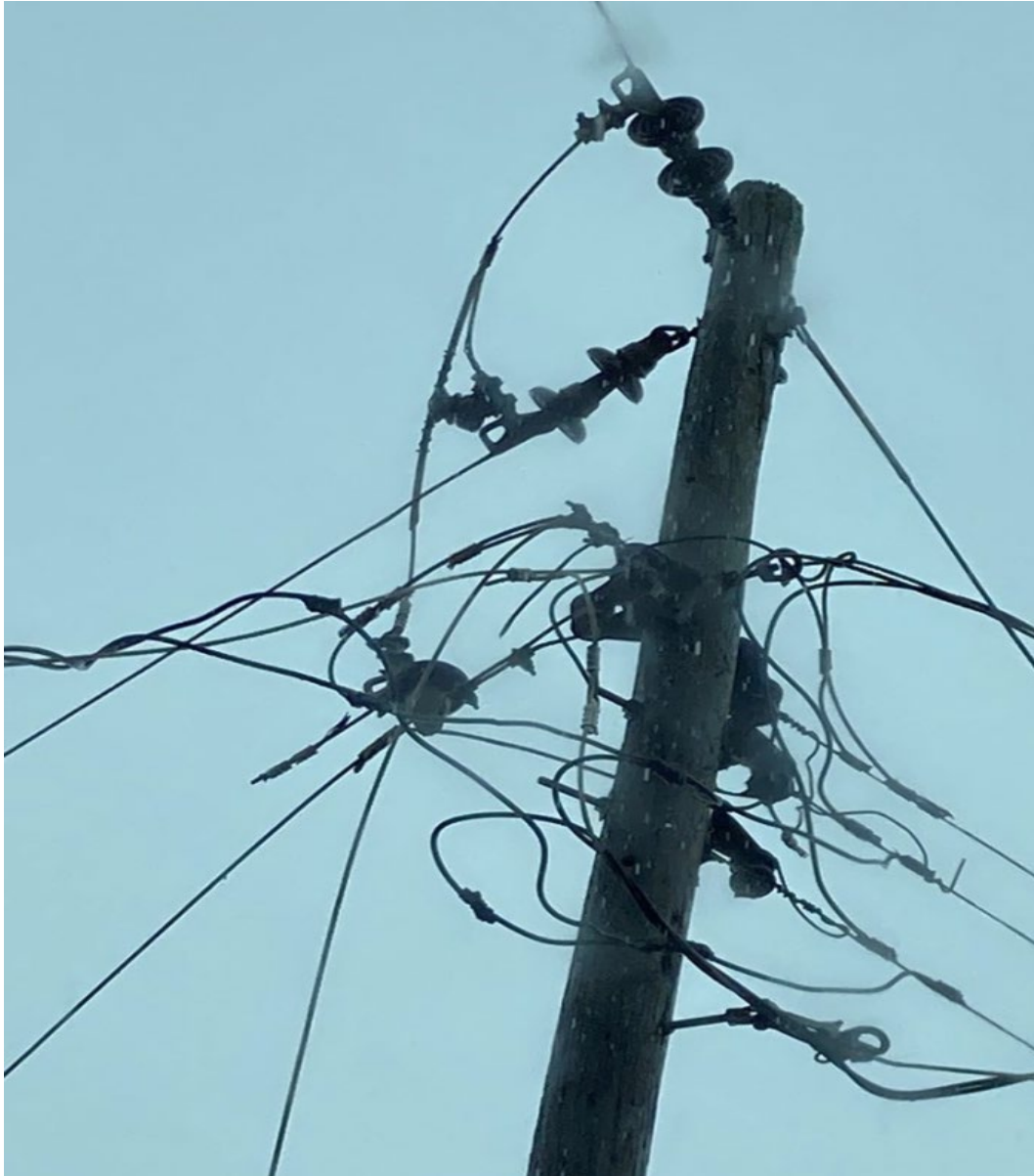
Insulator fail, broken hardware.
