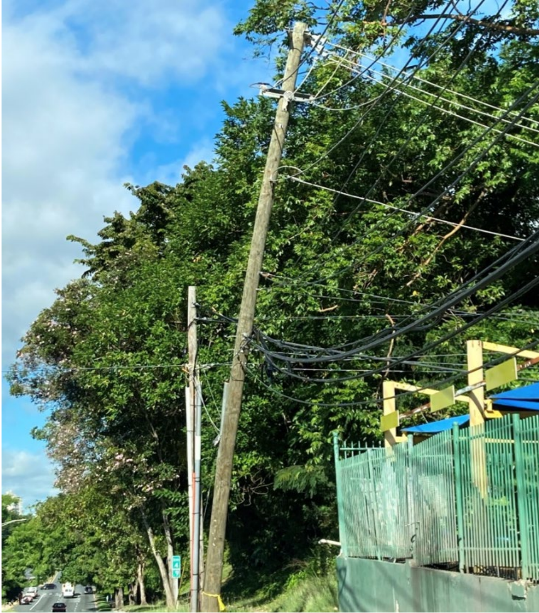
New pole installed incorrectly.
