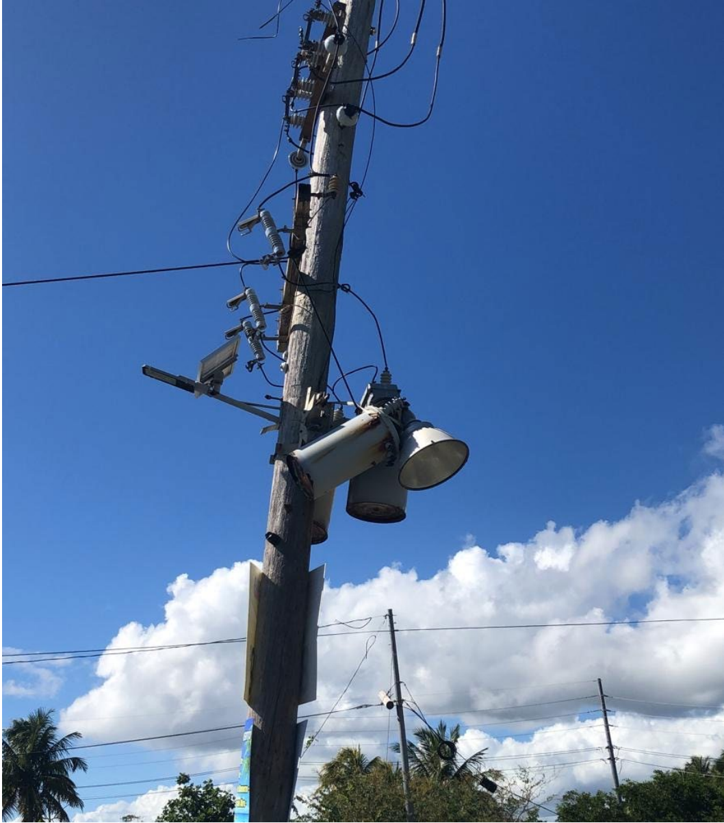
Transformer on light.
