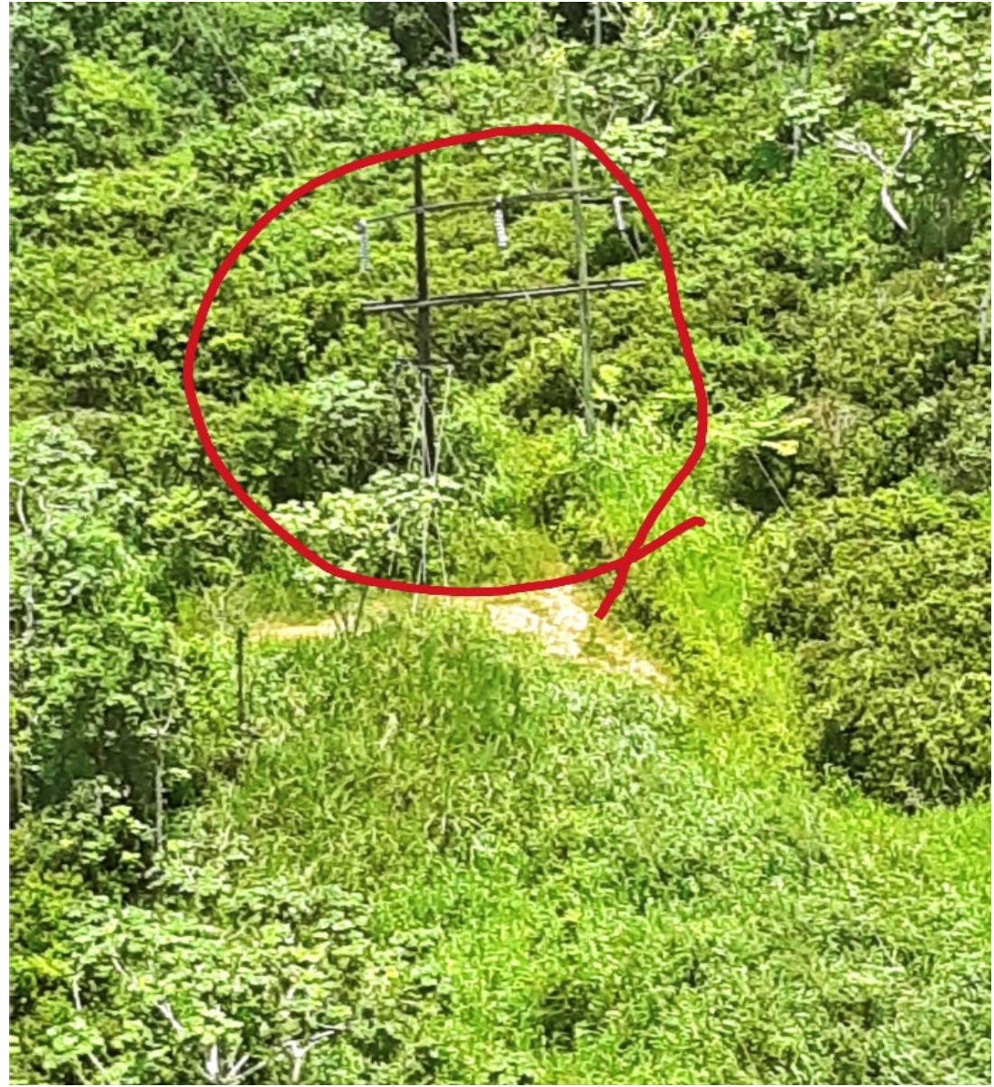
Tx line 36100 failed pole with circuit still on.
