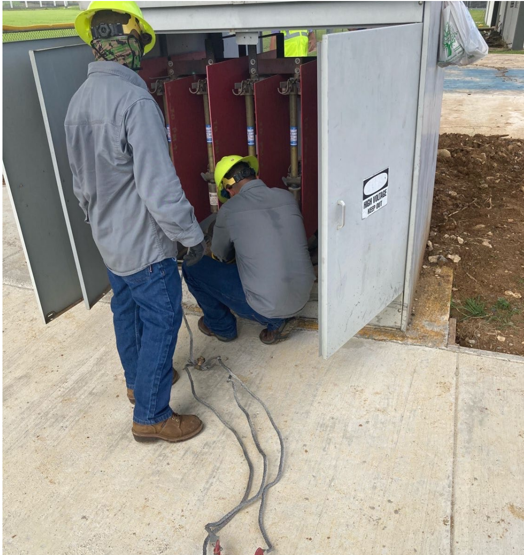
The phases were contacting each other, rubber coverup installed instead of repairing.
