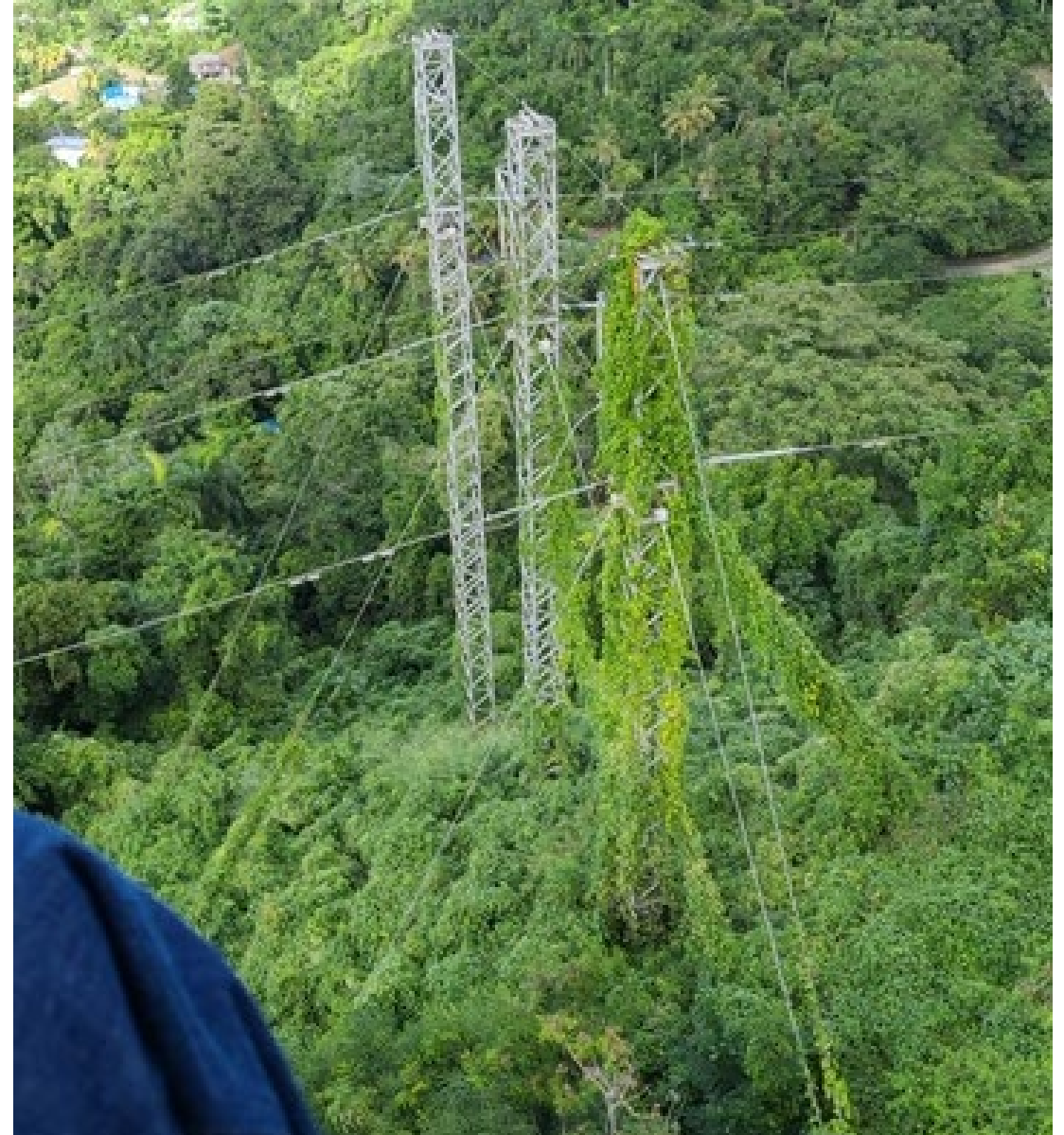
Heavy vegetation on transmission tower.
