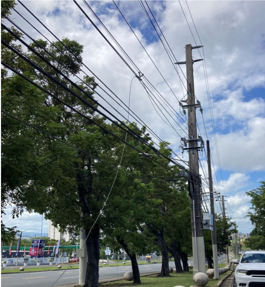
Damaged neutral conductor.
