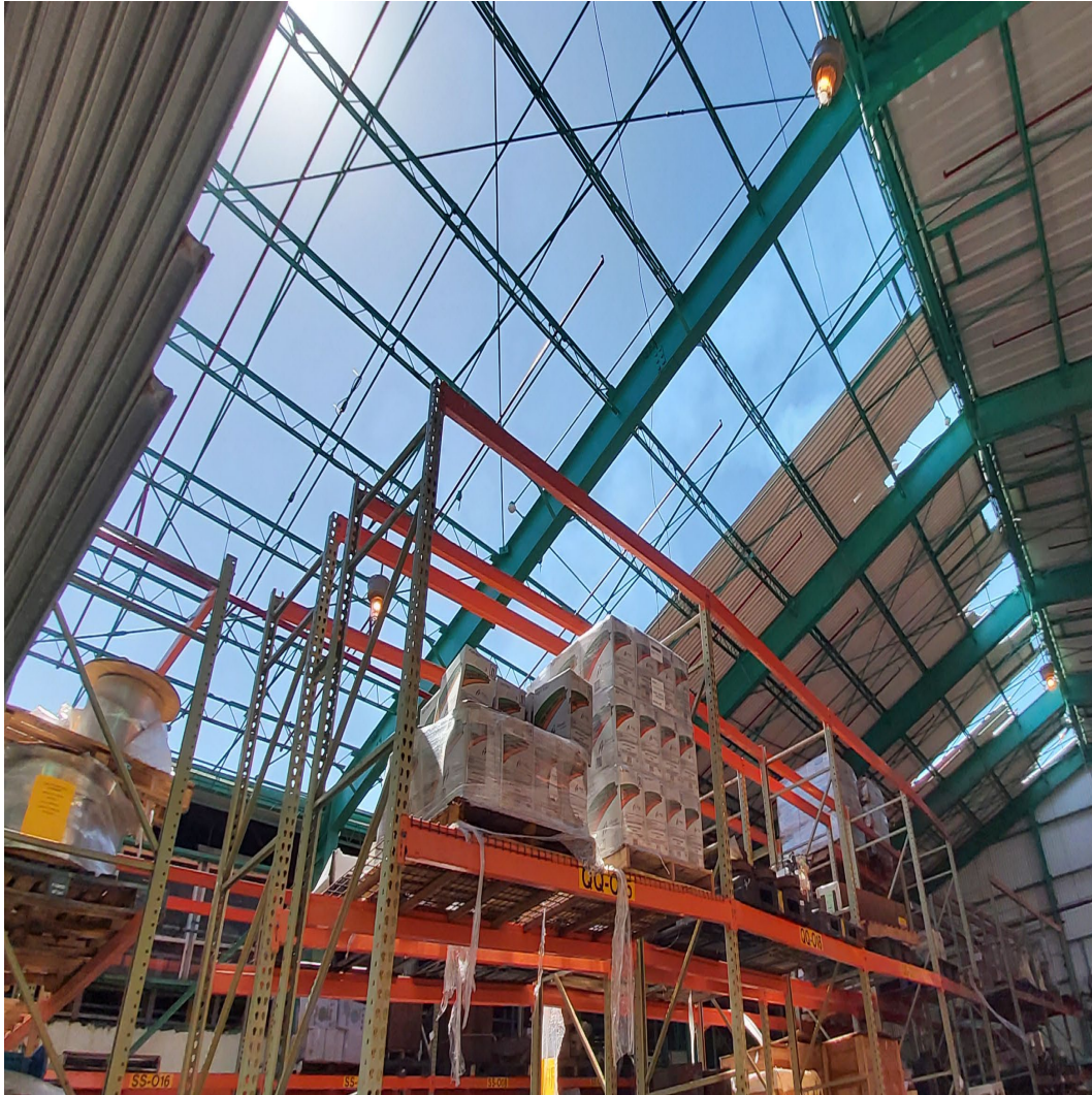
Aguirre Power Plant Warehouse. Roof missing since Maria, not prioritized causing heavy damage to material and racking from repeated rainfall.
