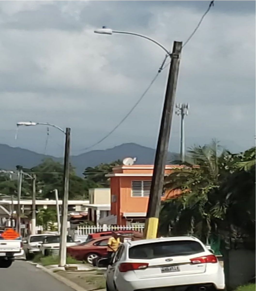
Primary wire suspended from streetlights.
