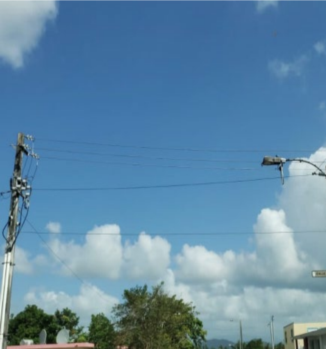
Primary wire ended on street light pole within limits of approach to primary line.
