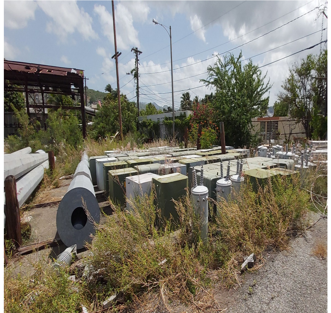
Yauco Yard. Non-stock Padmount Transformers 10+ years old.
