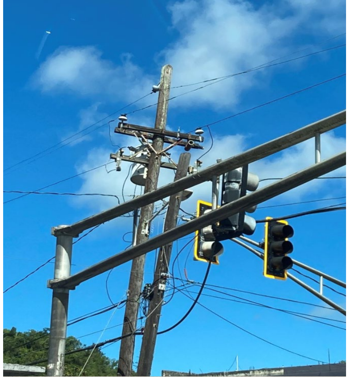
Hardware failure, wire against pole.
