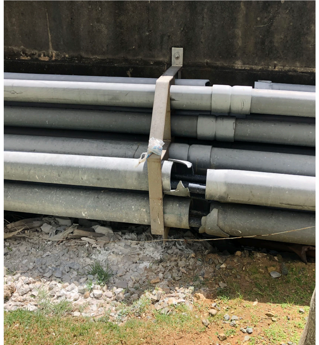
Failed primary underground cable.
