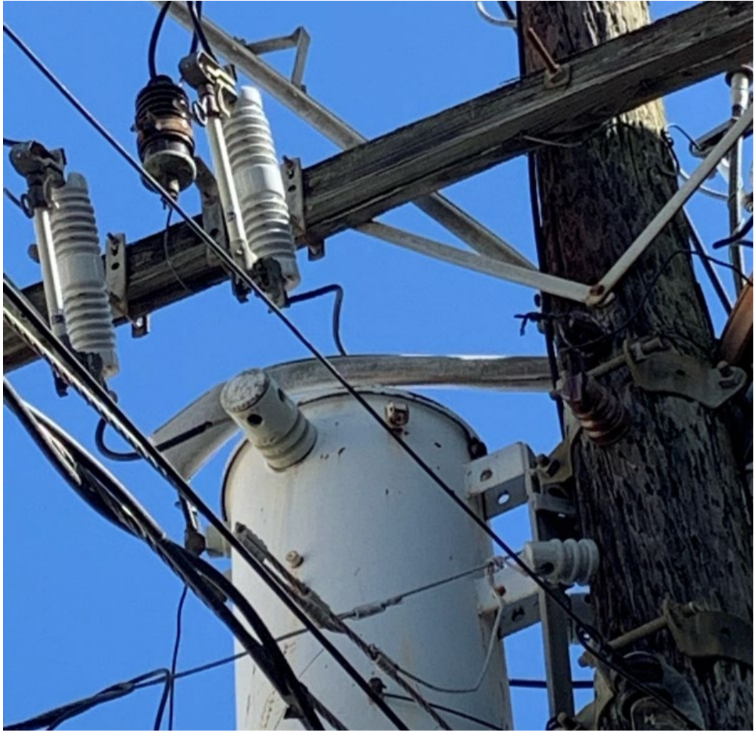
Primary conductor laying on top of transformer with line hose bleached white from sun exposure.
