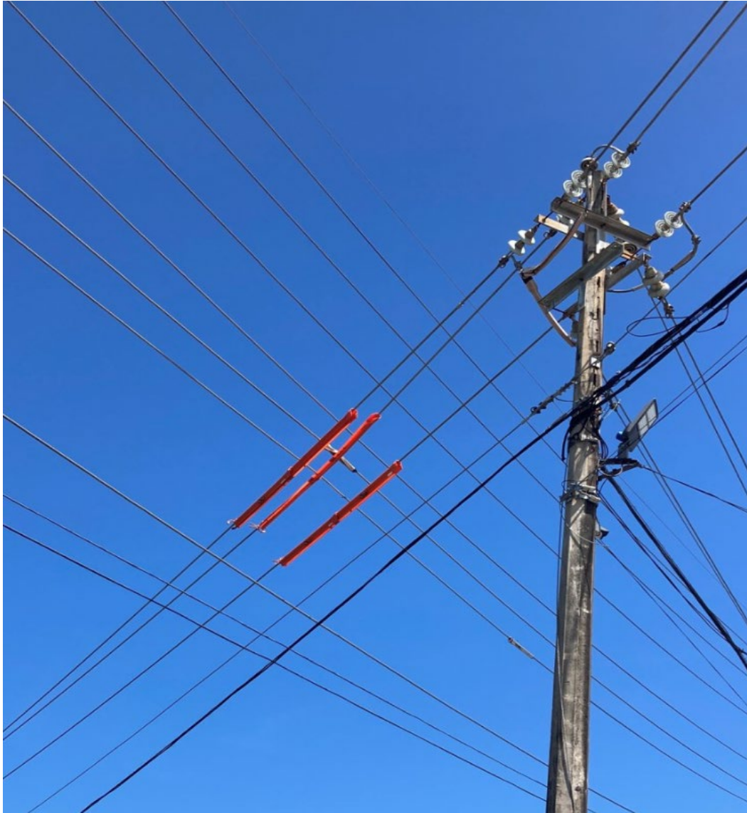
Primary Cable on Primary Cable - line coverup installed instead of repairing.
