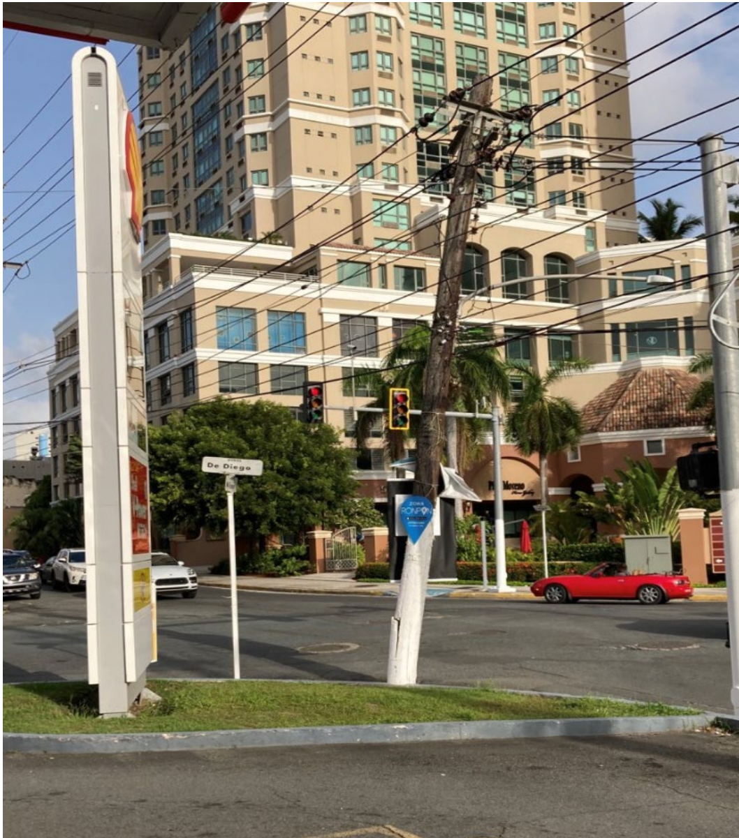
Pole crack at base.
