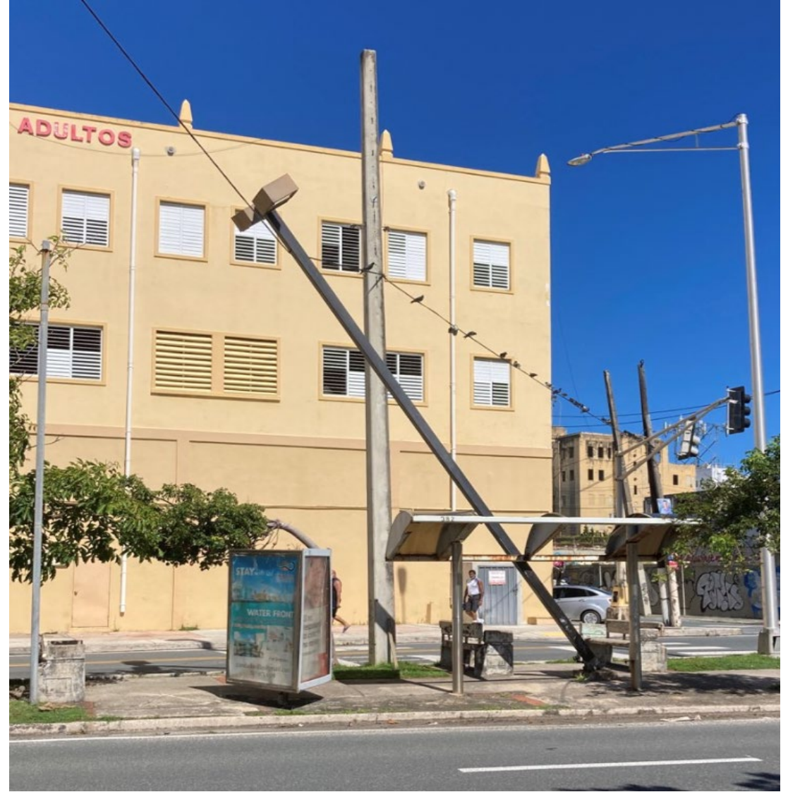
Failed streetlight pole on telecommunication cable.
