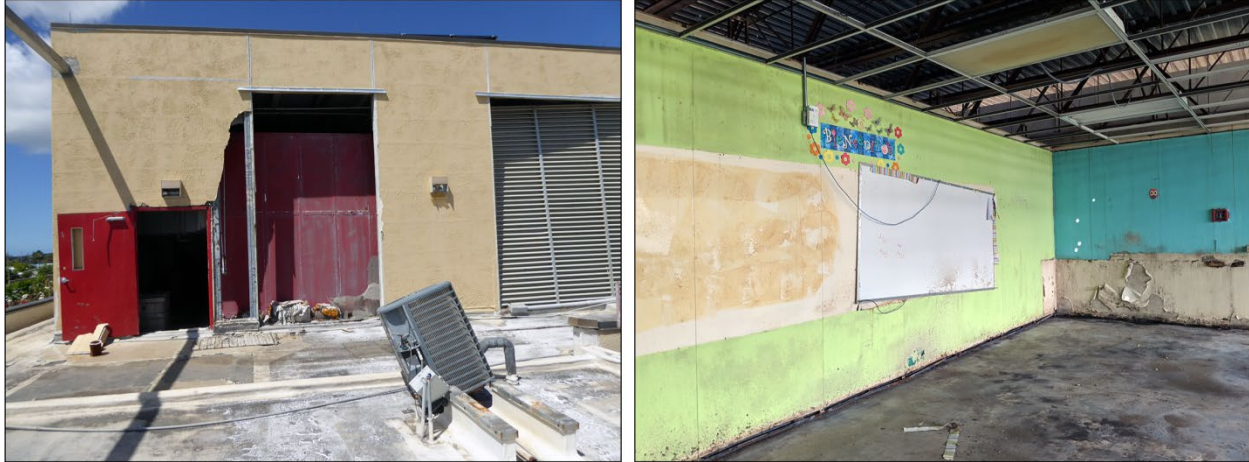
Damaged structure and ventilation system of the Governor Juan F. Luis Hospital and Medical Center in St. Croix, U.S. Virgin Islands.
