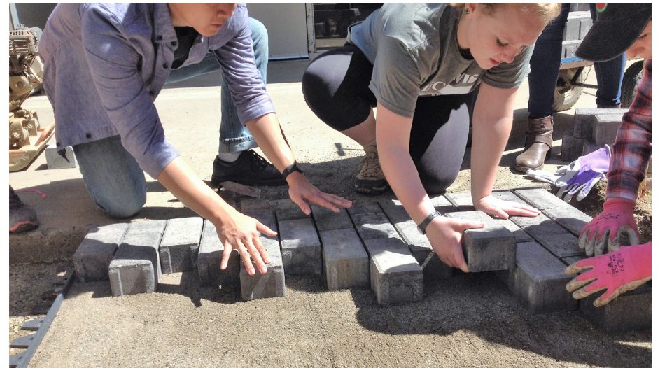
Students learn how to install an accessible pervious pavement pathway that runs through the Social Sciences and Humanities Rain Garden site. This new pathway now gives pedestrians the ability to easily move through the rain garden space without needing to walk through the previous eroded turfgrass condition.
