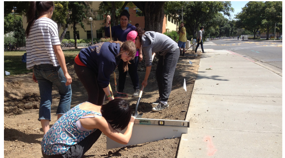
UC Davis students, many of which had never worked on a rain garden construction project before, learn how to shape the soil to allow stormwater to collect and slowly soak into our underground aquifers.
