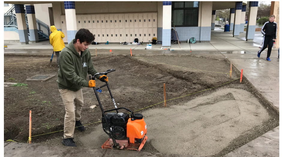
Davis High School students and the California Leadership in Green Infrastructure in the process of installation pervious paving that flank all sides of the new rain garden space.
