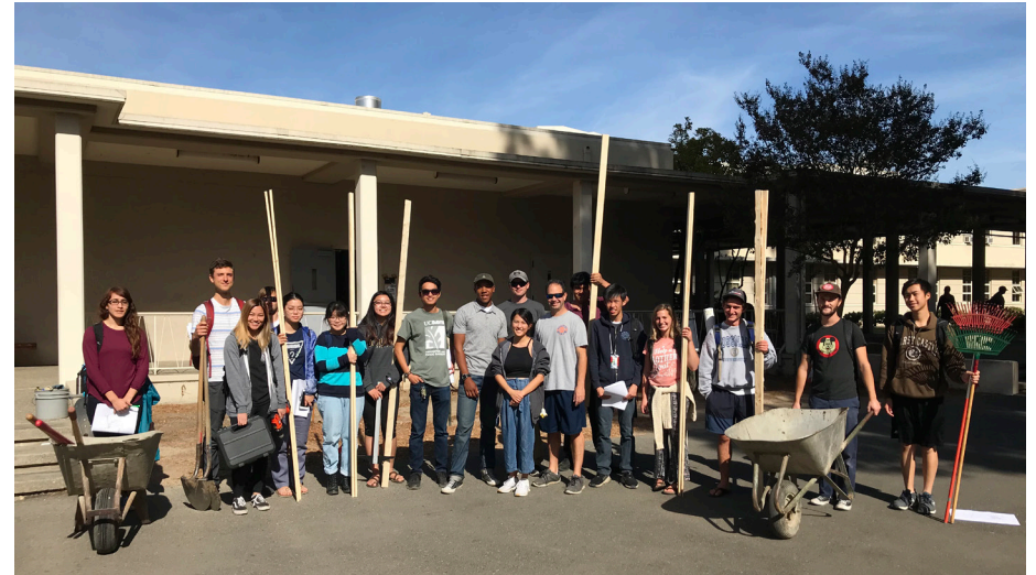
The October 26, 2018 groundbreaking for the Young Hall Rain Garden. Our multi-disciplinary student-practitioner team banded together to build our third campus retrofit and demonstrate the power of transforming underutilized spaces with Tactical Green Infrastructure.
