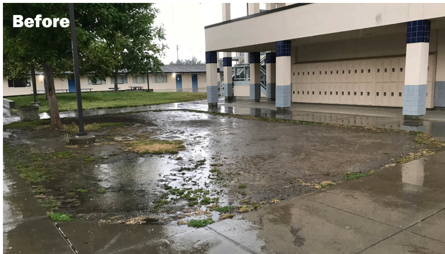
The highly visible existing courtyard space at Davis Senior High School was previously a highly compacted soil condition without any significant ground plane landscaping. During even mild rain events, this space would turn into a muddy mess and caused soil to be eroded and enter the piped storm drain system.
